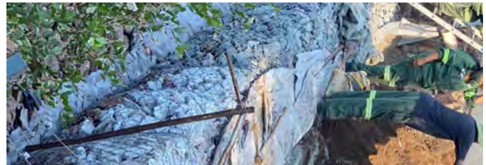
Repairs to bridge damaged by flood waters
