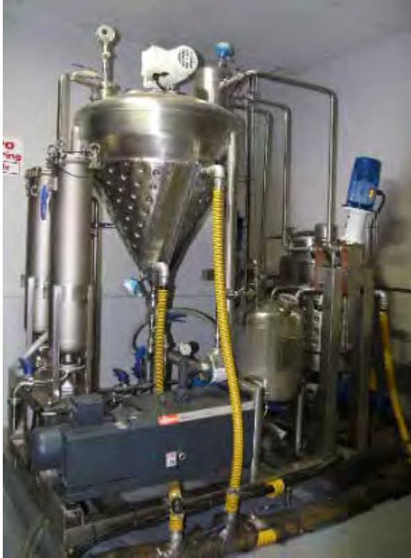
Figure 13: Ethylated fatty acid production plant
