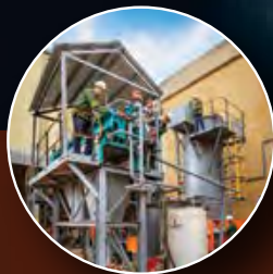
Water filtration plant is used to filter out solids in mineral processing
