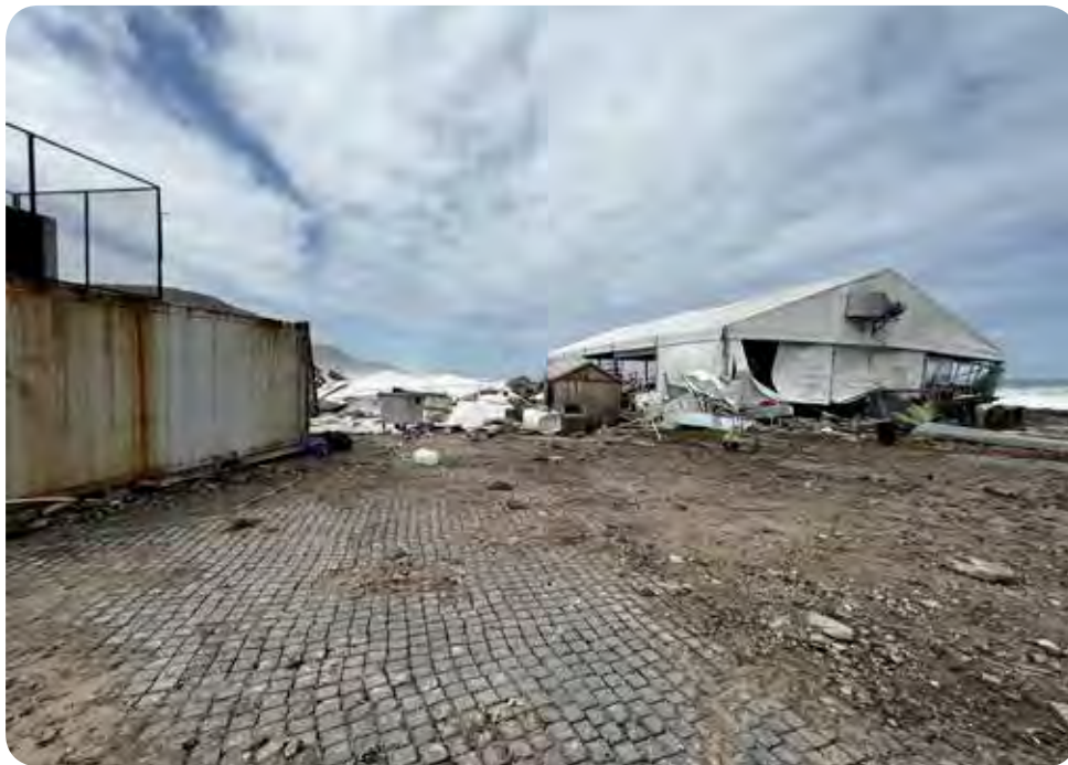
Severe damages to Tsitsikamma National Park's Cattle Baron restaurant due to the storm surge and spring high tides
