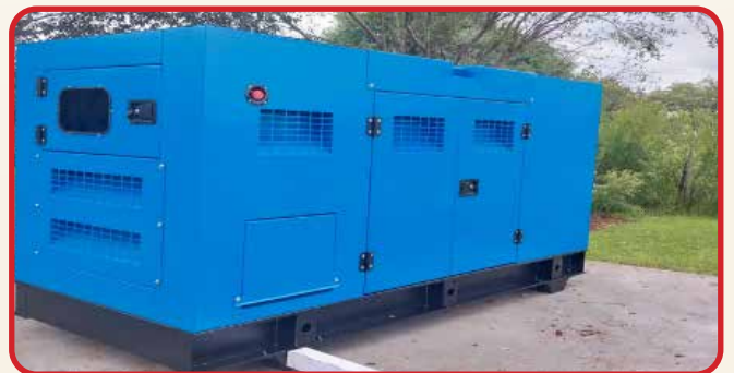
AP -New Generator.
