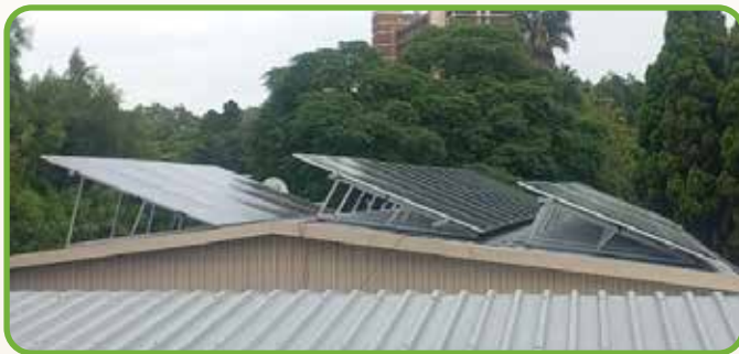
Solar Solution at NRE
